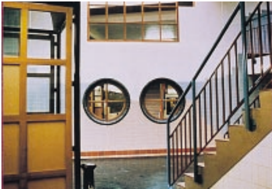
Top - Housing Estate Stairwell subject to severe graffiti abuse Bottom - Subsequent refurbishment using Armourlac
